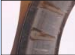
Etching, considerable corrosion.
