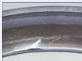
Damaged by spindle
